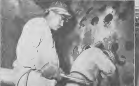
EVERYTHING GETS a careful going-over from valves to pumps. The convection section, left, its tubes pulled, is shown being cut up by workers. That face plate, right, will be lifted off by a derrick and the tube bundle inside pulled as part of the project to increase the visbreaker's efficiency of operating. About 320 men are involved.
